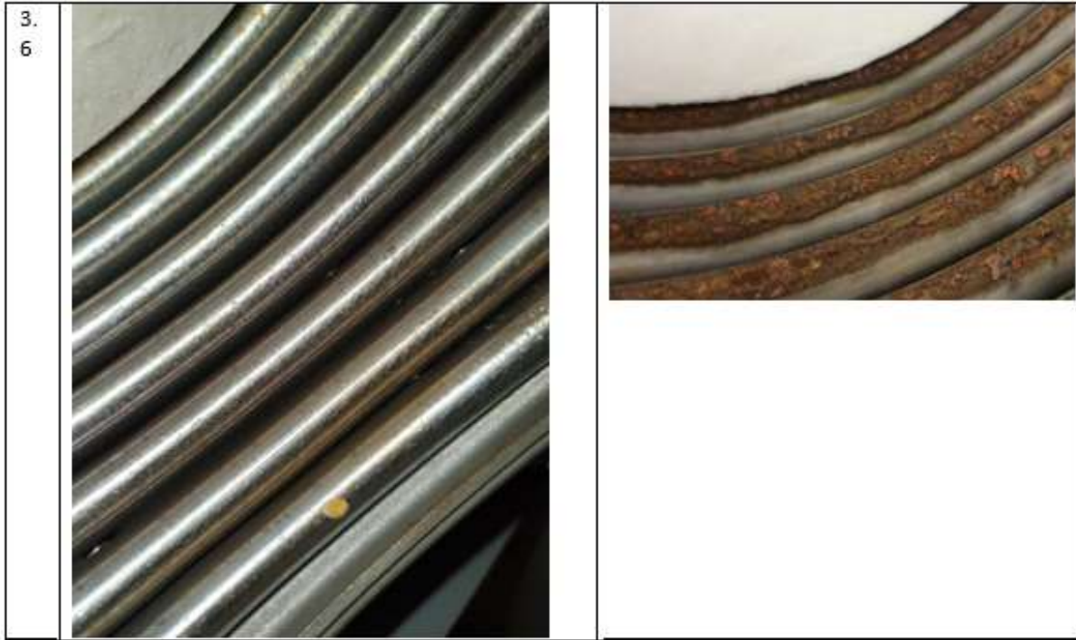
Figure 23: Pictures of boiler 3 (D6)
