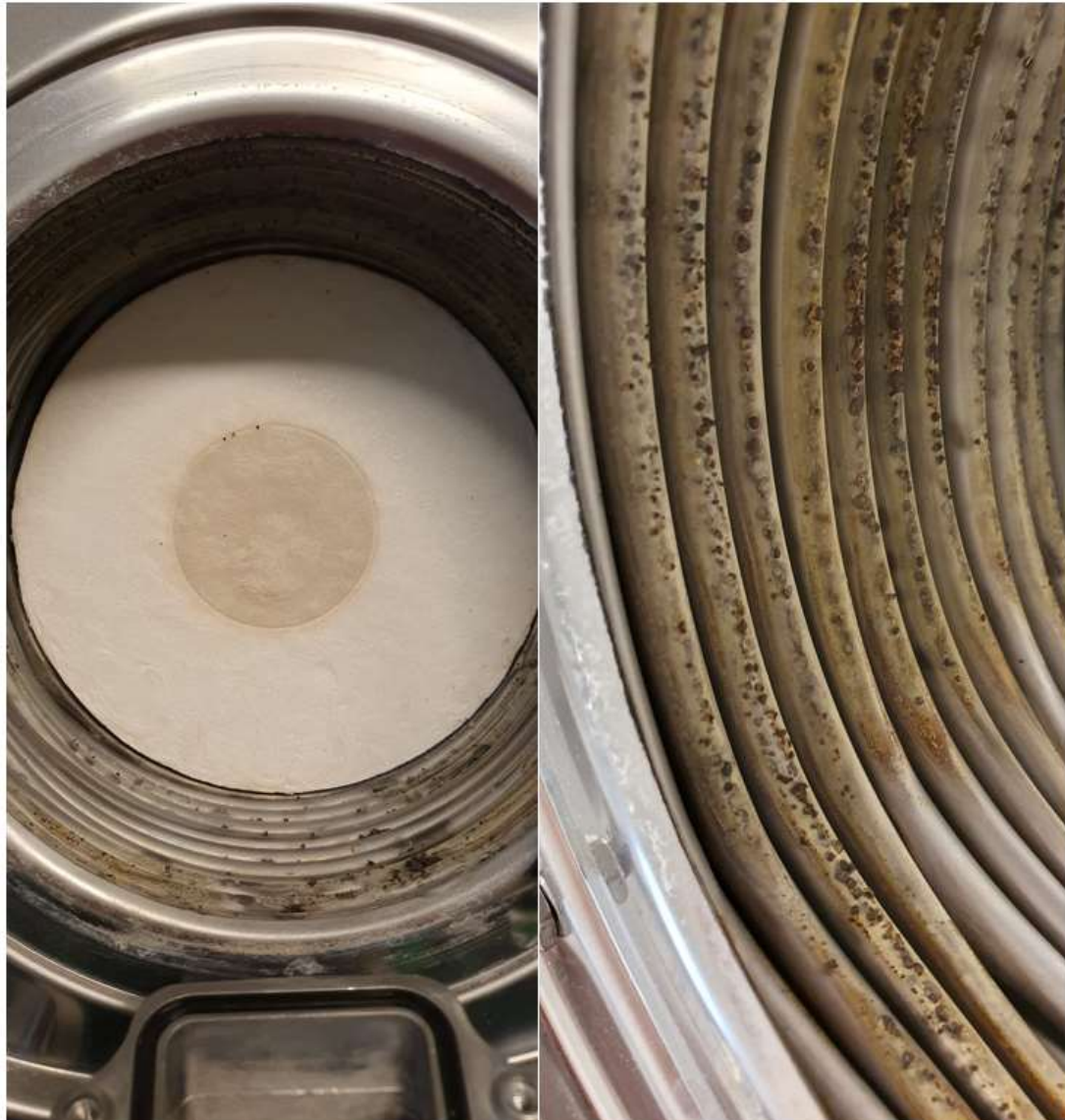
Figure 17: Front and closeup view of boiler 1 heat exchanger (D4)
