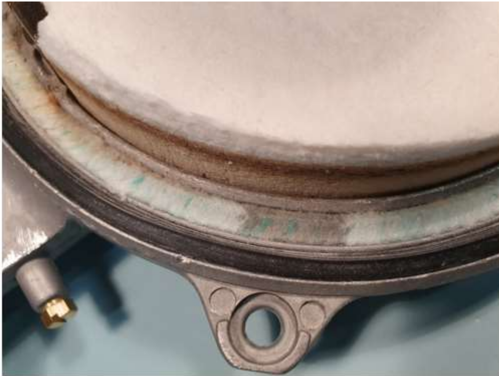
Figure 22: Closeup of isolation of boiler 2 (D5)
