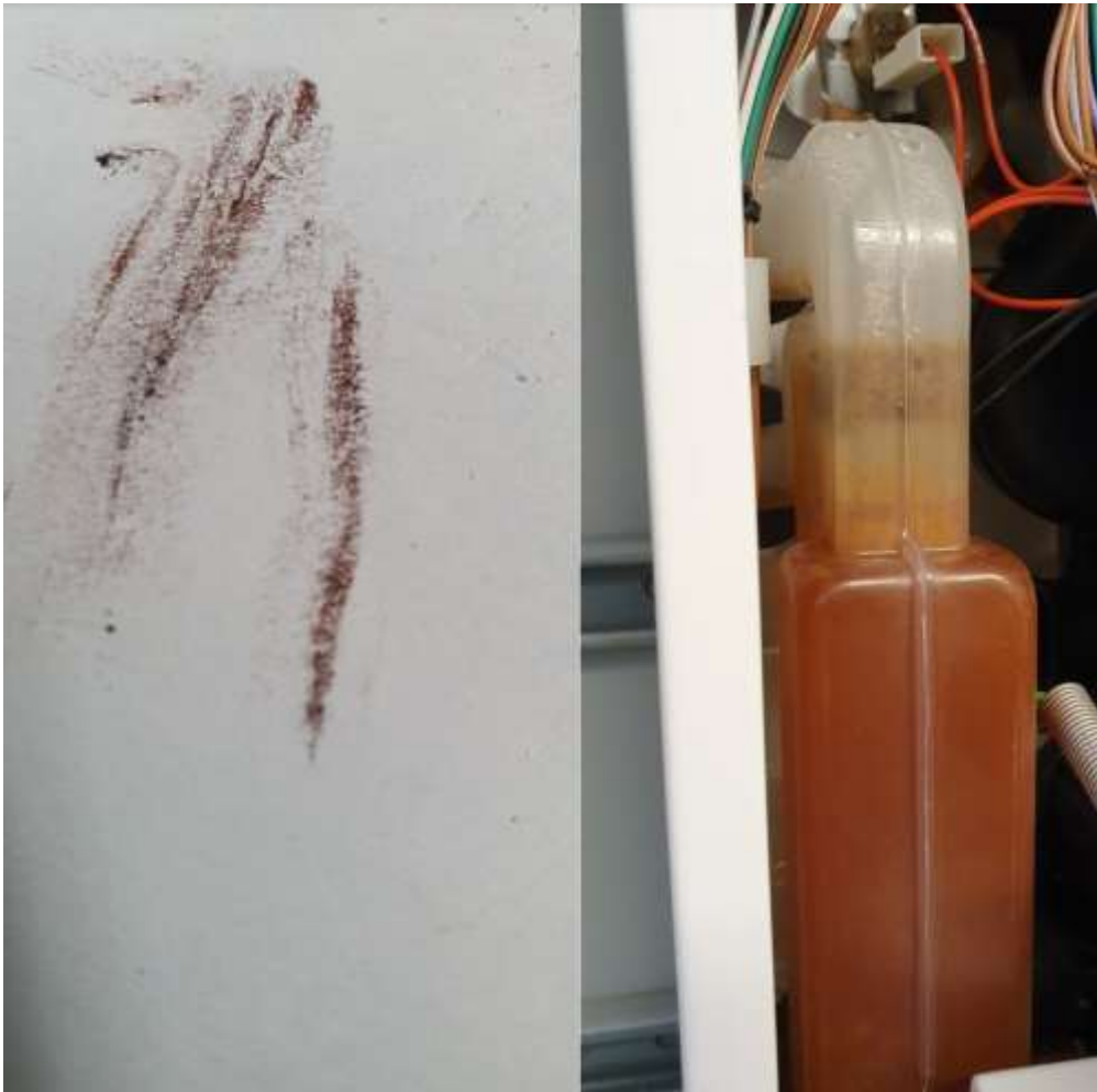
Figure 19: Deposit in boiler 1 (D4) spread on paper on the left, deposit in the boiler (“condensate reservoir”) on the right.
