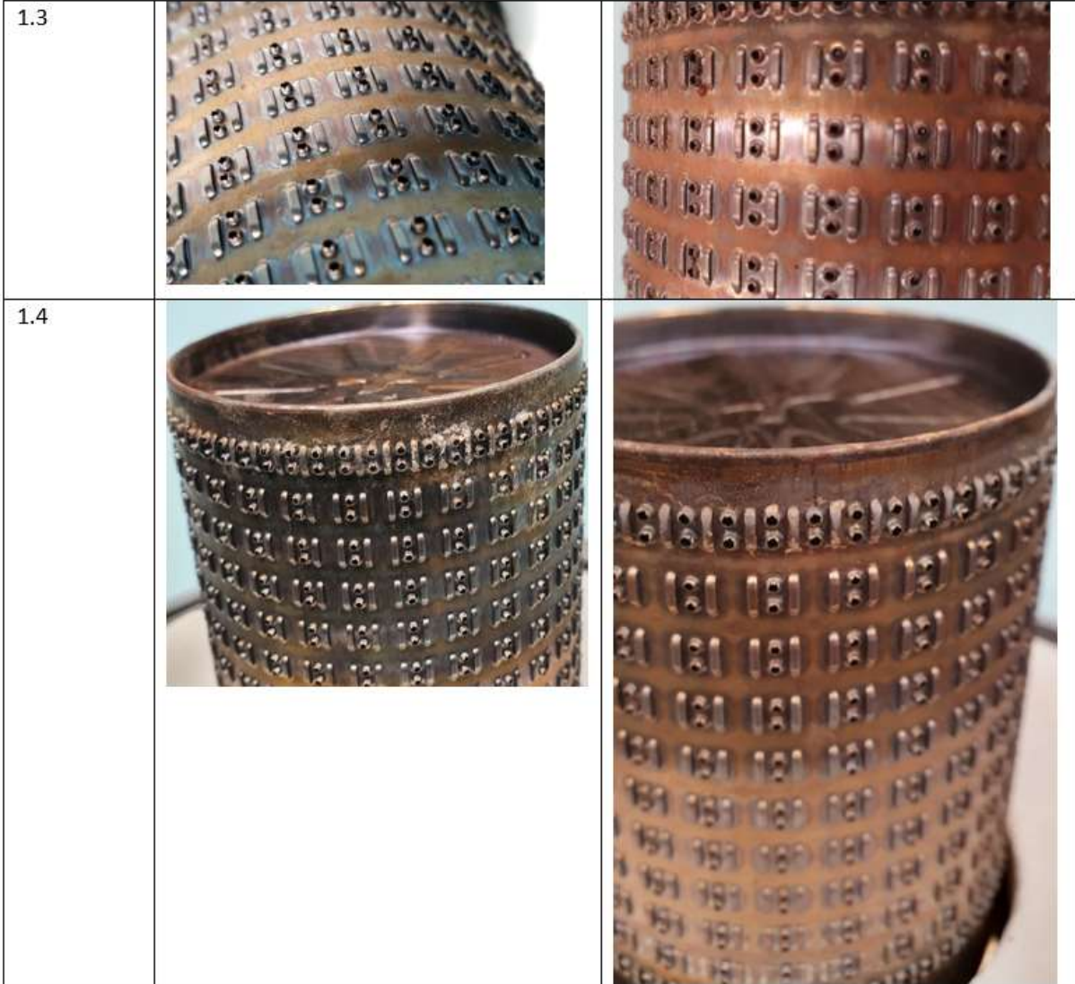
Figure 16: Pictures of boiler 1 Burner (D4)
