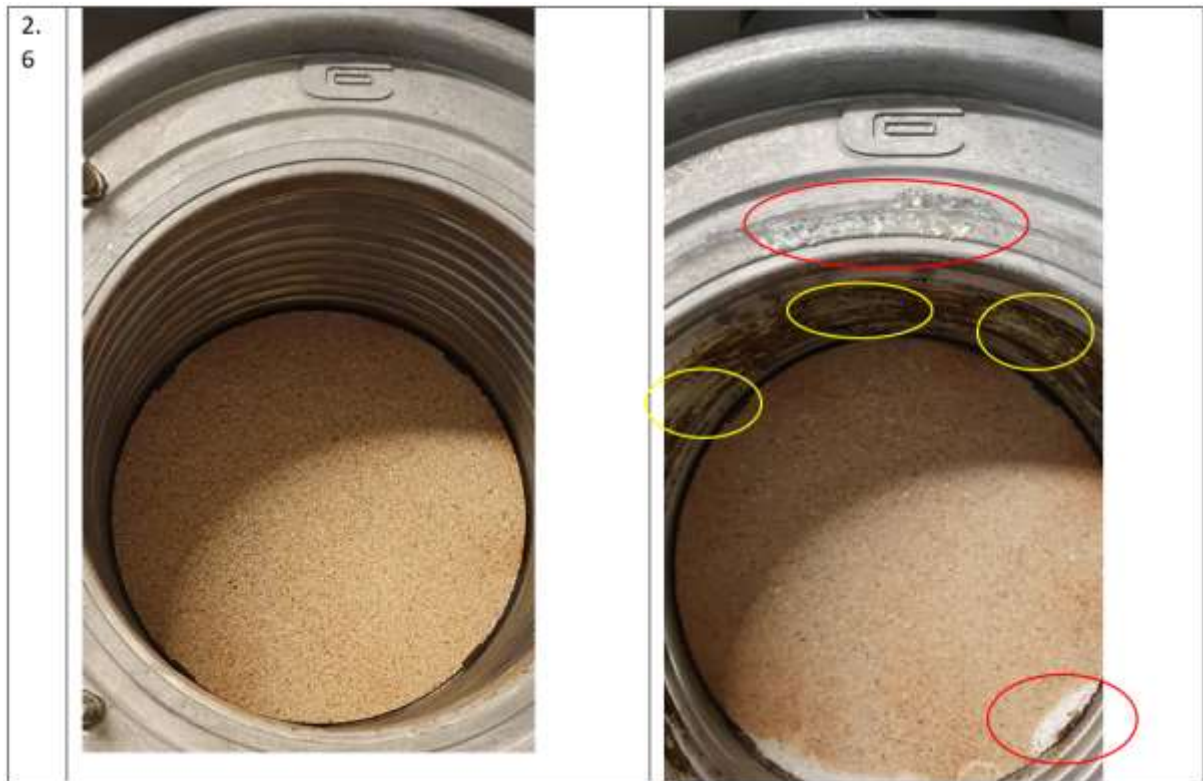
Figure 20: Pictures of boiler 2 (D5)
