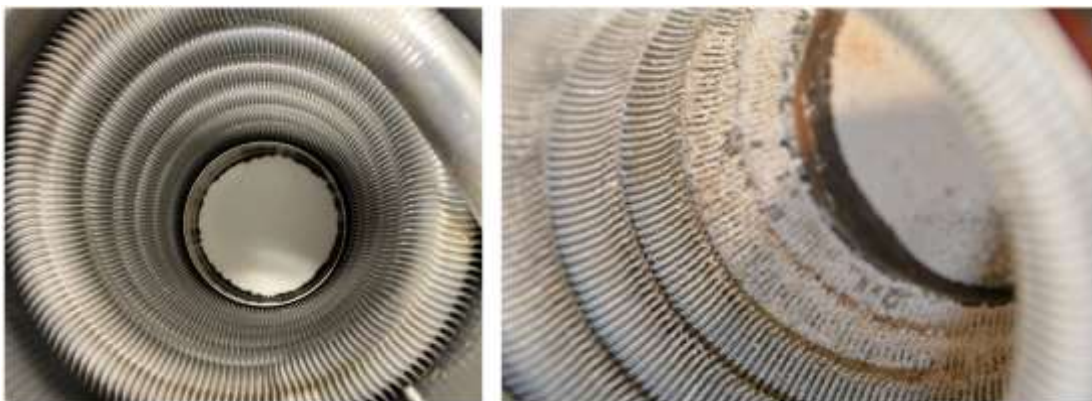
Figure 5: Boiler 2 – Heat exchanger before (left) and after (right) long term test. The observed deposits correspond to typical natural gas operation.
